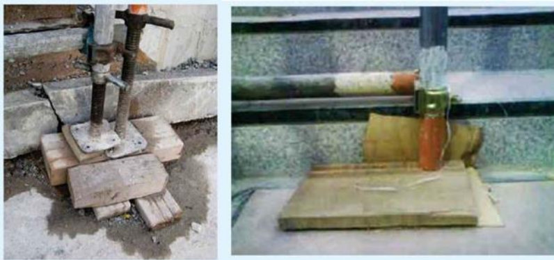
Scaffolding installed onto an unstable base
