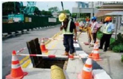
The entrance supervisor keeps track of workers and monitors the people working inside the confined space
