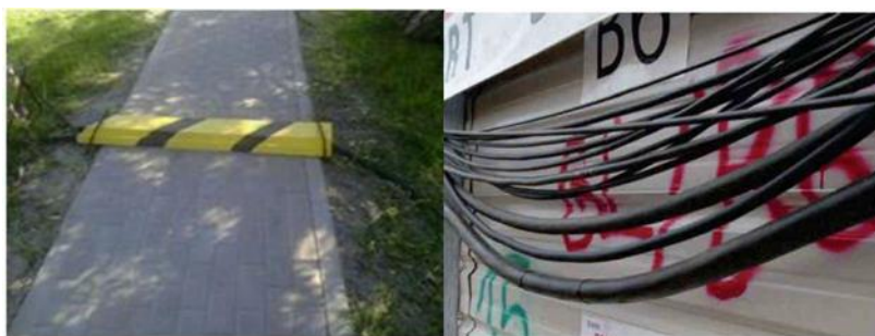
Covered or elevated cables in traffic areas
