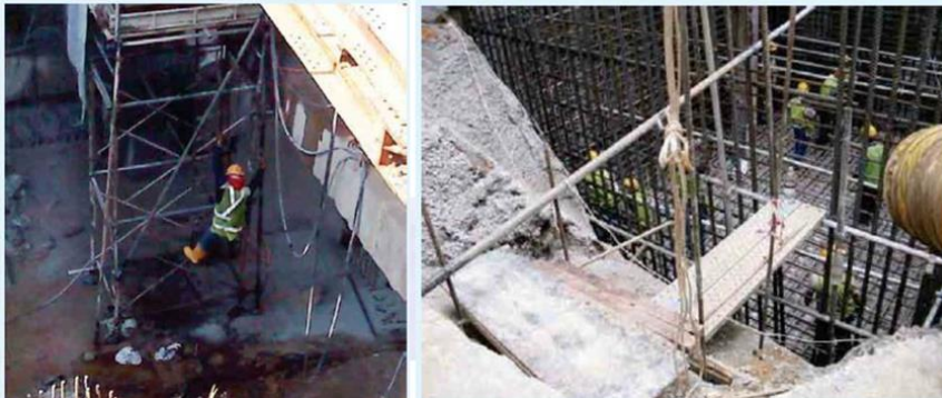
Unsafe access and moving around scaffolding
