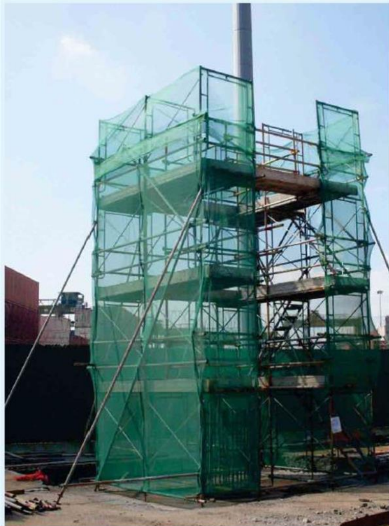
Side supports installed on scaffolding, and there is a way to move safely from one level to another
