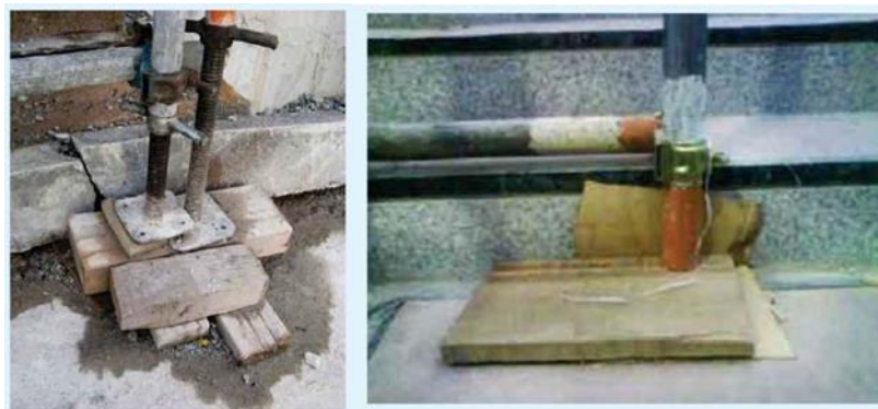
Scaffolding installed onto an unstable base
