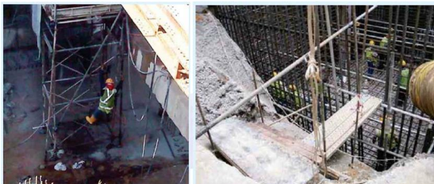
Unsafe access and moving around scaffolding
