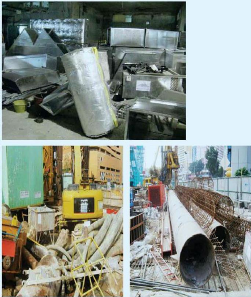
Improper placement and storage of materials
